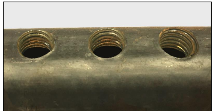
FIGURE 6: Unacceptable Rust in Coupler Threads
