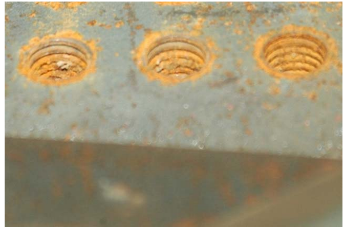
Figure 5. Unacceptable Rust in Coupler Threads
