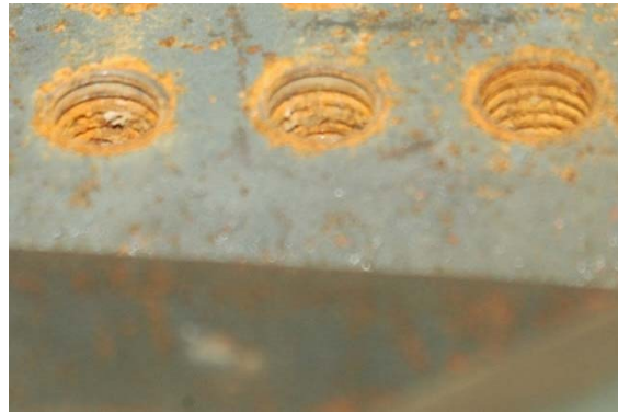
Figure 5. Unacceptable Rust in Coupler Threads
