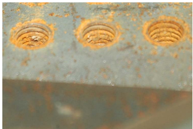
Figure 6. Unacceptable Rust in Coupler Threads
