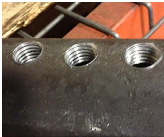
Figure 5. Clean Acceptable Coupler
