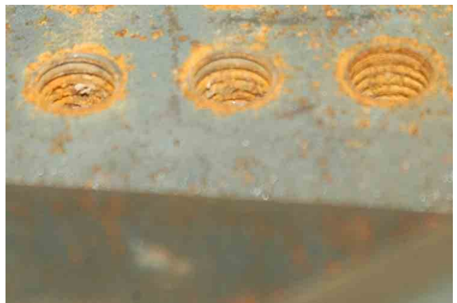
Figure 6. Unacceptable Rust in Coupler Threads
