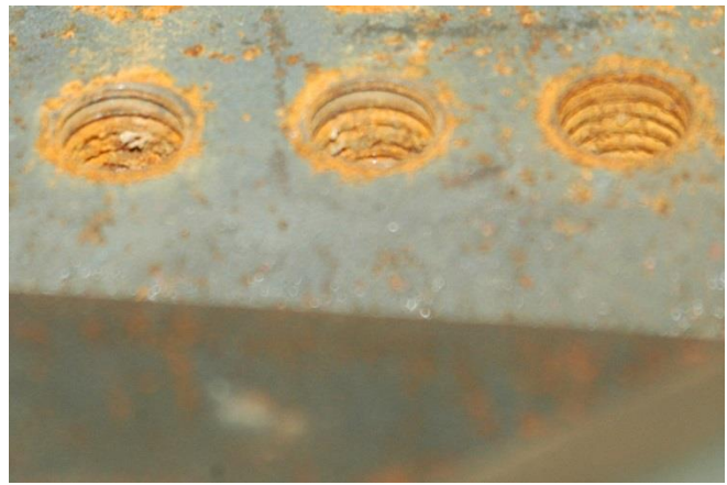
Figure 7. Unacceptable Rust in Coupler Threads
