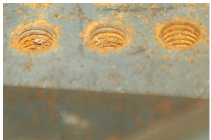
Figure 6. Unacceptable Rust in Coupler Threads
