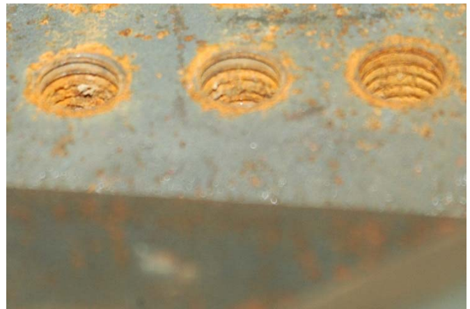
Figure 6. Unacceptable Rust in Coupler Threads
