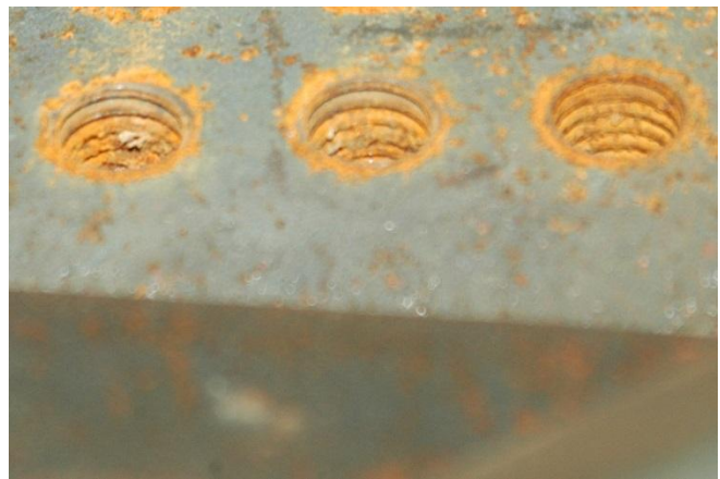
Figure 7. Unacceptable Rust in Coupler Threads
