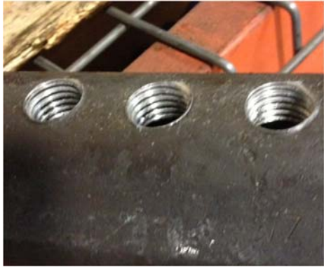
Figure 4. Clean Acceptable Coupler
