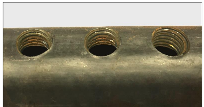
FIGURE 6: Unacceptable Rust in Coupler Threads
