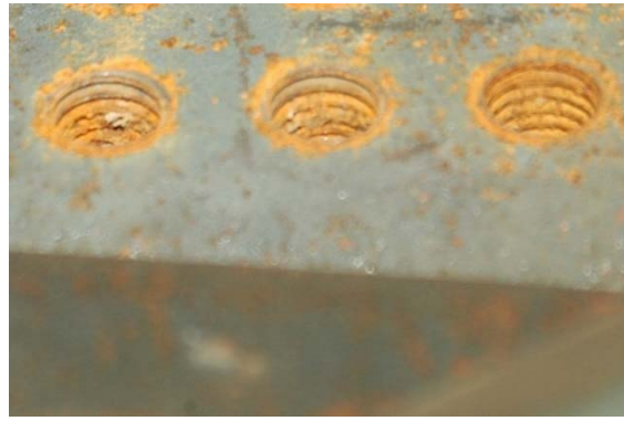
Figure 5. Unacceptable Rust in Coupler Threads
