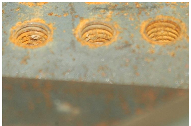
Figure 6. Unacceptable Rust in Coupler Threads
